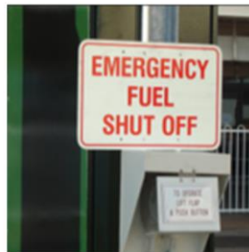
Emergency Fuel Shut Off Button
