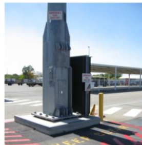
Apron lighting pole
